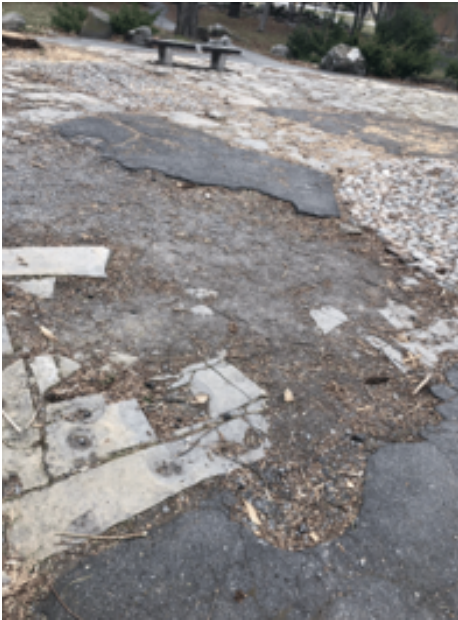
Figure 2: Decorative stone surface destroyed by winter plowing and tree root encroachment
